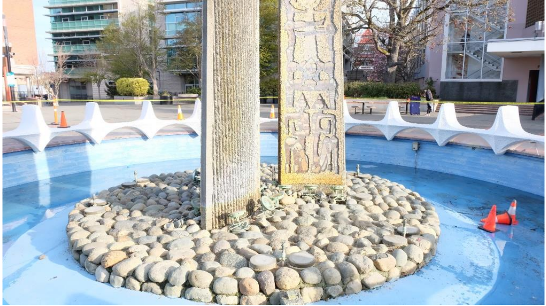
Examination of the base was conducted down to base level of the structures.
