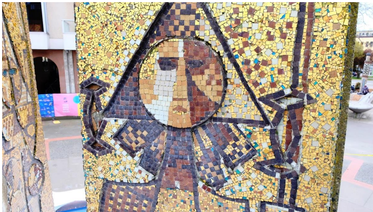
Impact damage to tiles noted in this photo.
