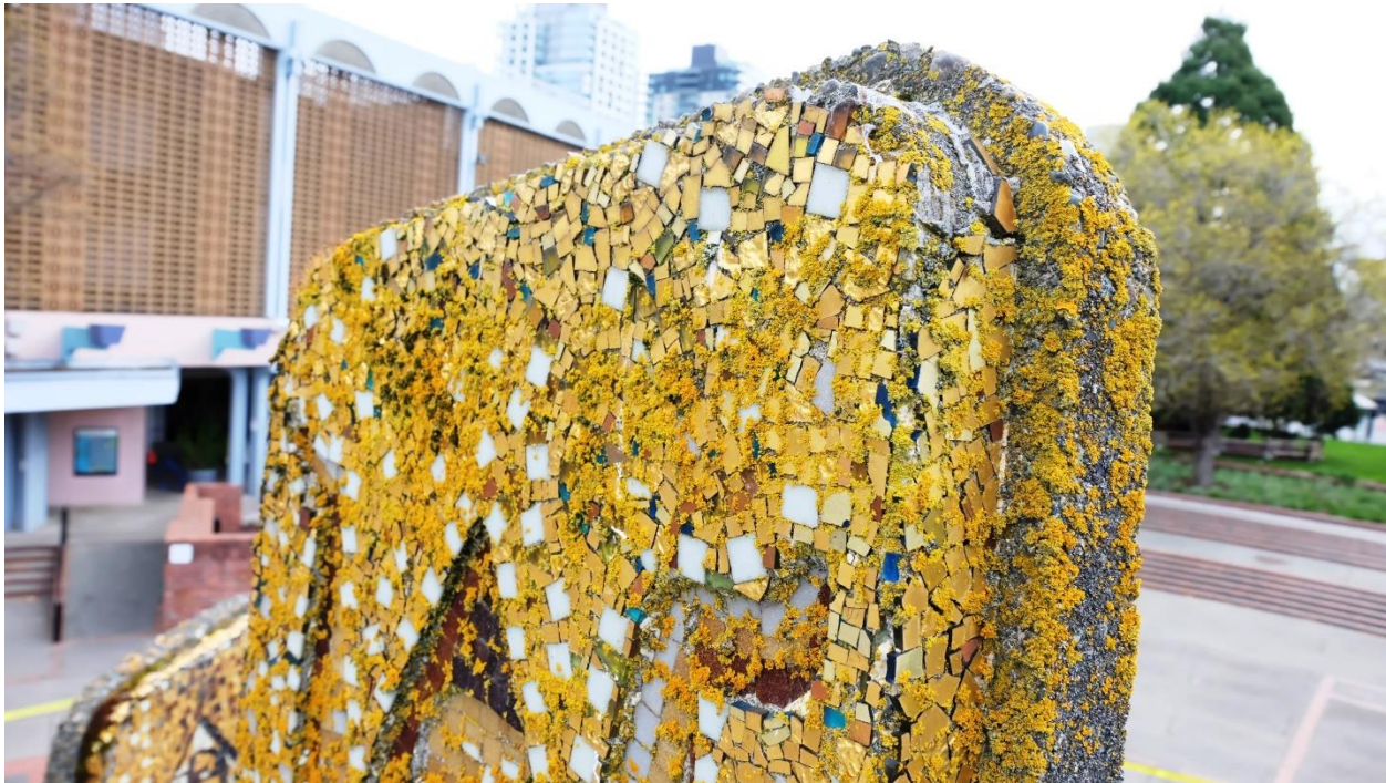
Examination of the upper surfaces found conditions of heavy moss/lichen fungal growths
